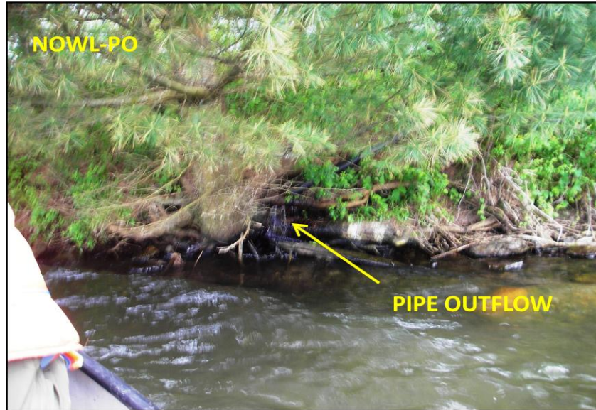
Fig. 4.2.3 Pipe outflow along the lower eastern shoreline of Nowlans Lake.
